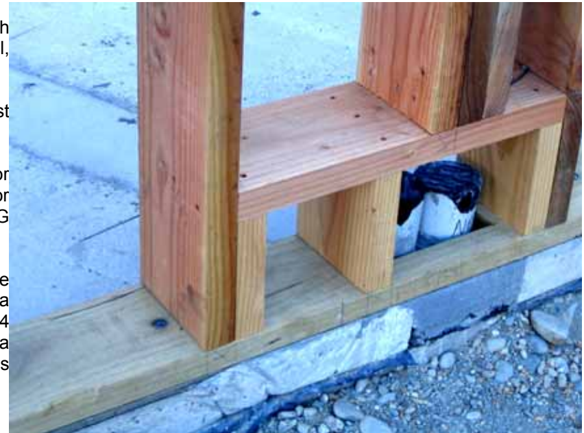
Untreated Douglas Fir used as framing. In this case treated Radiata is used for the bottom plate.
