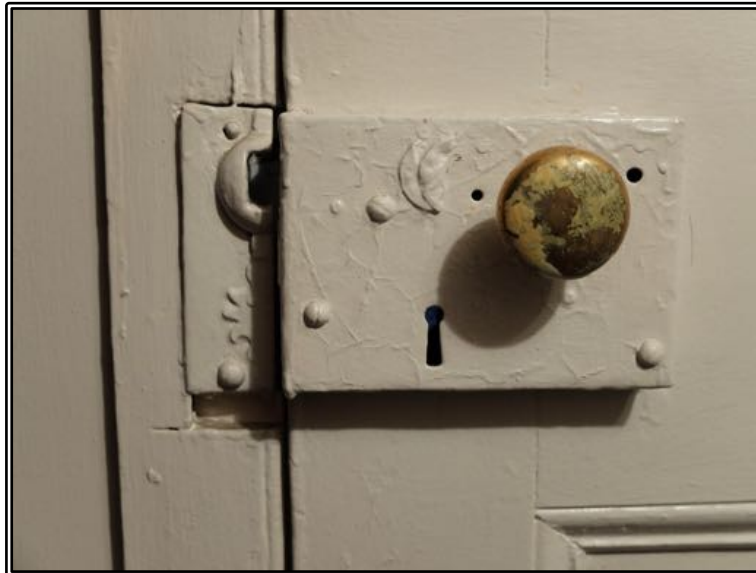
Figure 30 The lock on the bathroom door.
