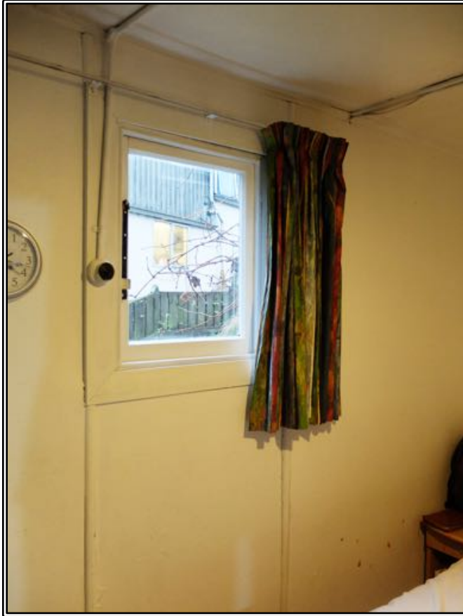
Figure 25 The side wall of the bedroom, with the twentieth century casement window.
