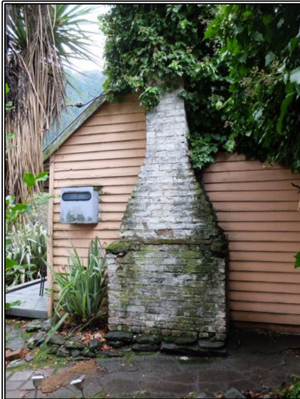
Figure 15 The south wall of the cottage, showing the brick chimney and creepers.
