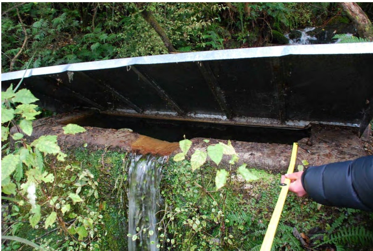
Photo 5 The concrete storage tank (approx. 200mm thick walls) with rudimentary overflow.
