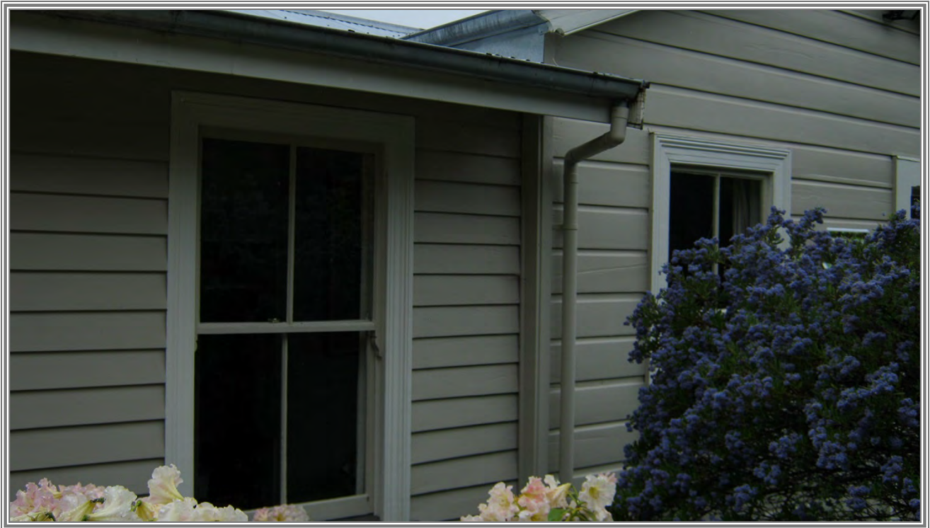
Fig. 1, Showing the original feather edge juxtaposed with the newer scallop rusticated weatherboard
