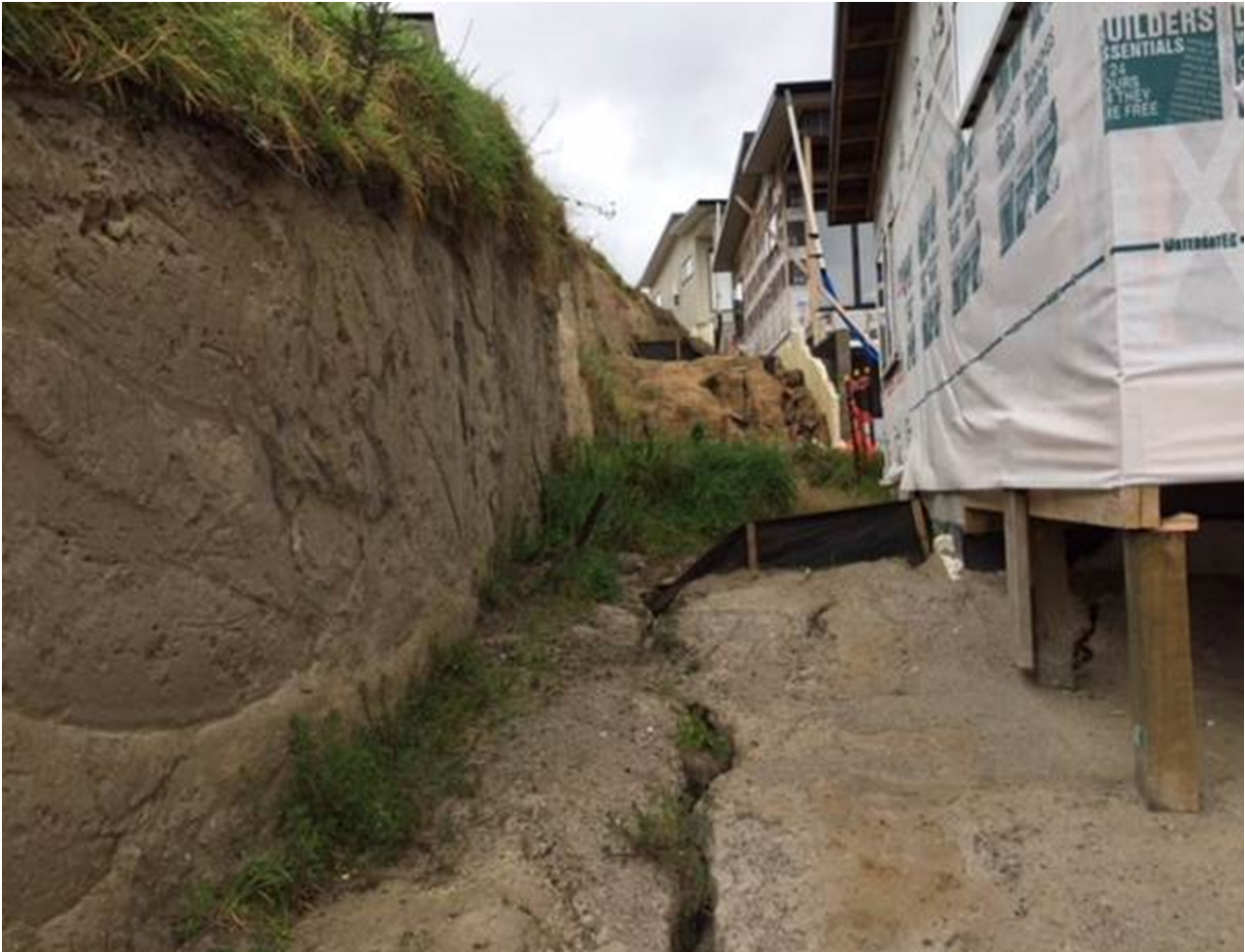
Figure 6: Example of an unretained cut along a property boundary of the Bella Vista Development.
