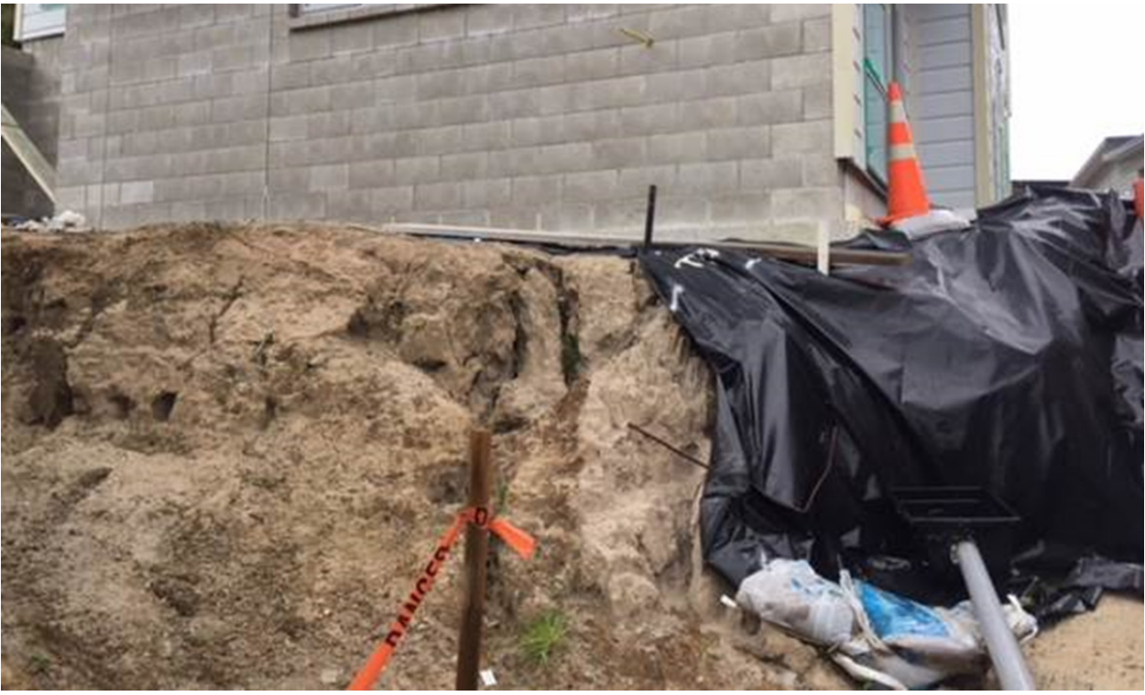
Figure 4: Unretained section of soil which provides support to a dwellings external masonry wall
