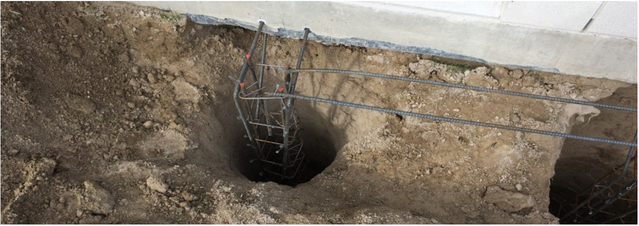
Figure 9: Foundation underpinning at an Aneta Way property. This was treated as a minor variation, but should have been processed as a formal amendment to the building consent.
