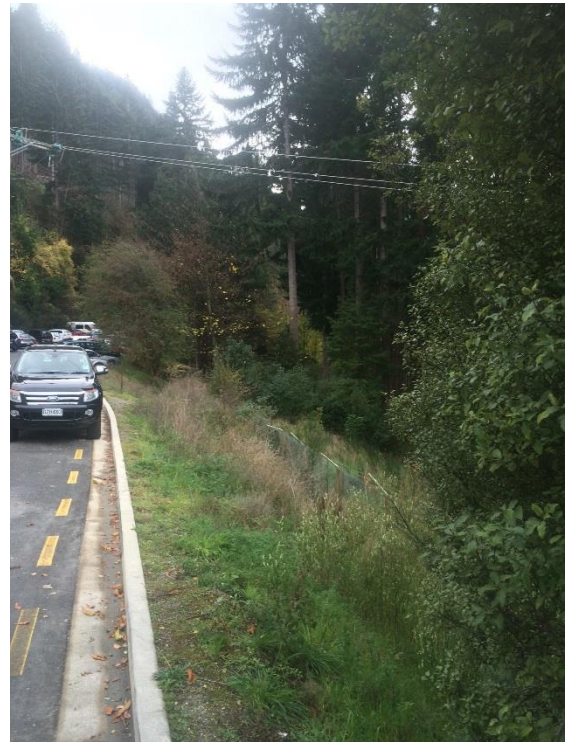
Photograph 4. Unkempt Steep Grass Embankment within Lot 2 DP 345184 looking North from Section 1 SO 22971.
