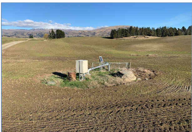
Photo 10: Water pump, west of the waste disposal area.
