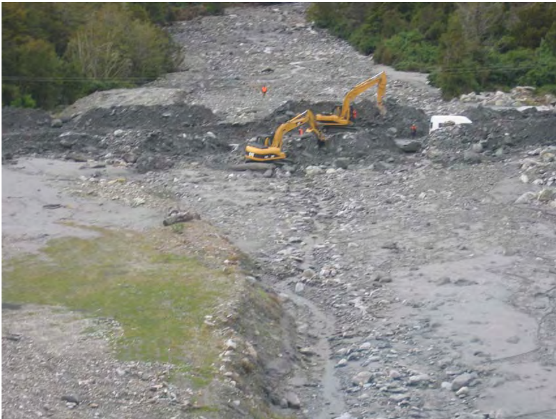
Figure 26: SH6 at Pipson Creek, showing debris from the 2006 event.
