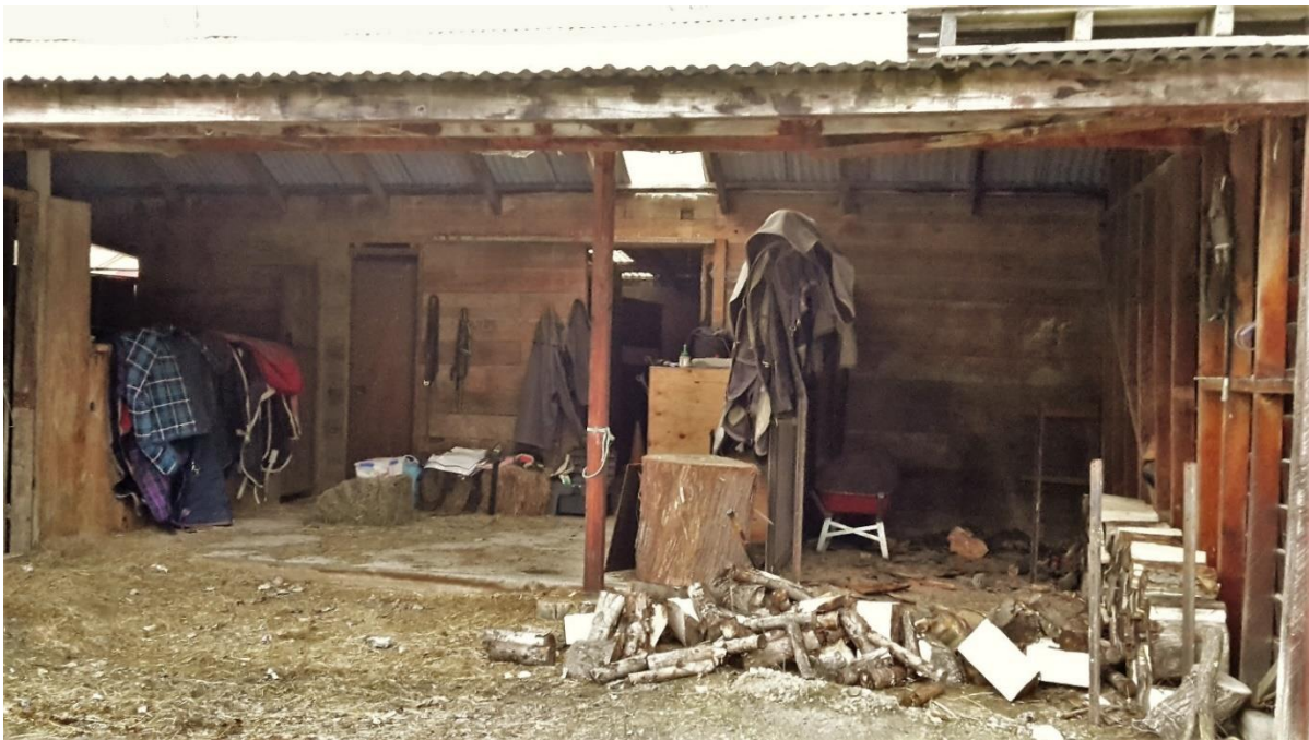
Figure 19: Interior of Shed/Stables showing equestrian equipment and general condition of shed interior.
