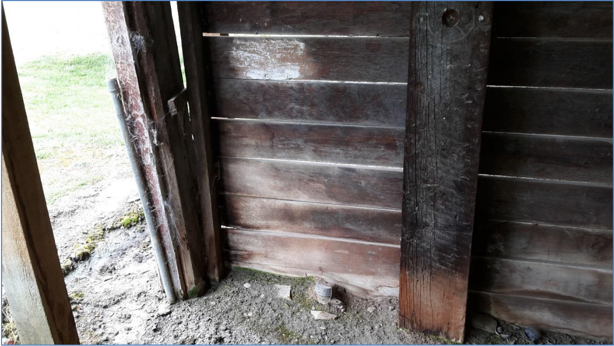
Figure 25: Fill point, tank breather and mounting point for pump against an internal wall in the Old Implement Shed, all serving as indicators of the presence of a second UST at site.
