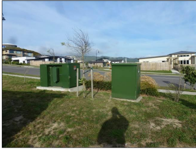
Figure 5: 300kVA Distribution Transformer with Adjacent Ring Main Unit
