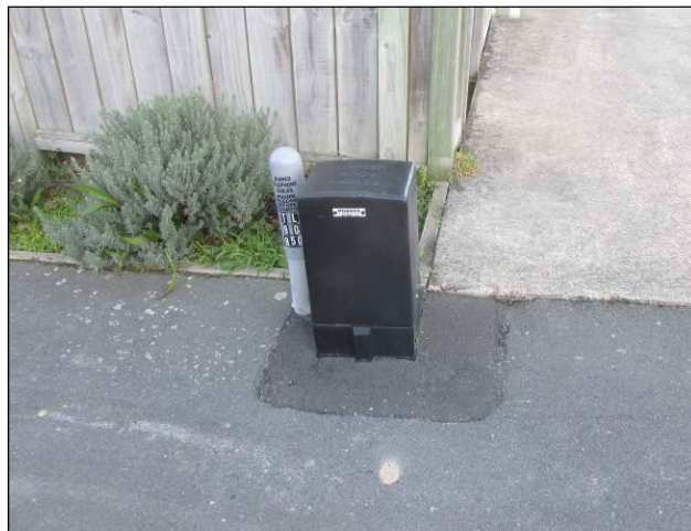
Figure 1: Typical Service Fuse Box
