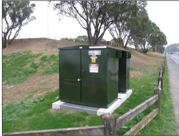
Figure 6: Typical Compact Substation incorporating Transformer and Ring Main Unit
