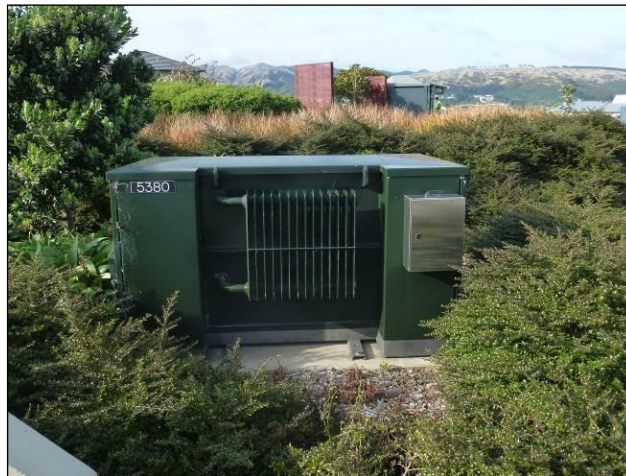
Figure 4: Typical 300kVA Distribution Transformer
