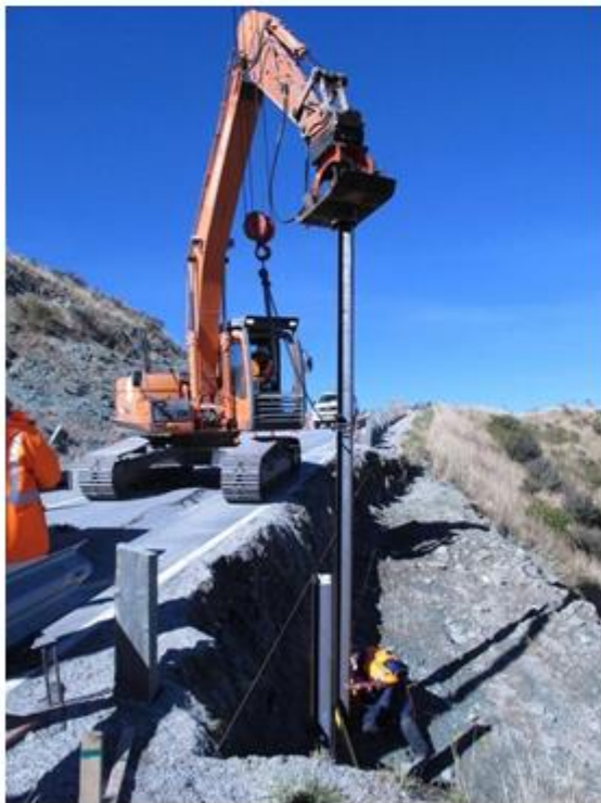
Figure 5. Pile driving at site 2 during construction 11 years ago, showing the length of the piles. The working shelf has completely disappeared.
