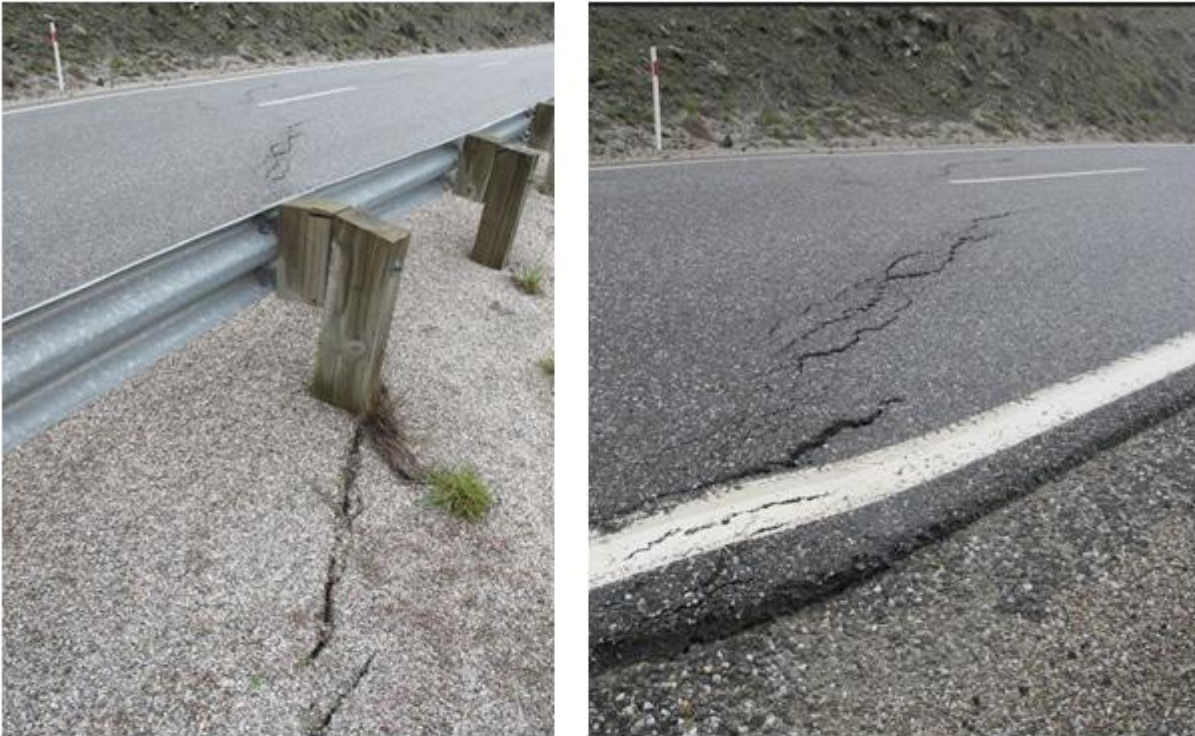
Figure 10. 50mm settlement in the pavement at site 3
