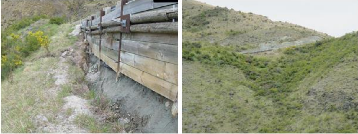
Figure 4. Site 2 with slope failing and sliding away from toe of retaining wall.
