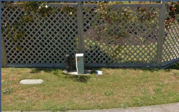
Telecommunications Pillar (pale green)
