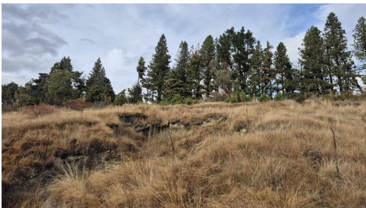
Photo 5.1 – Photo showing the erosion scouring below the water race on the southern side of the central depression.
