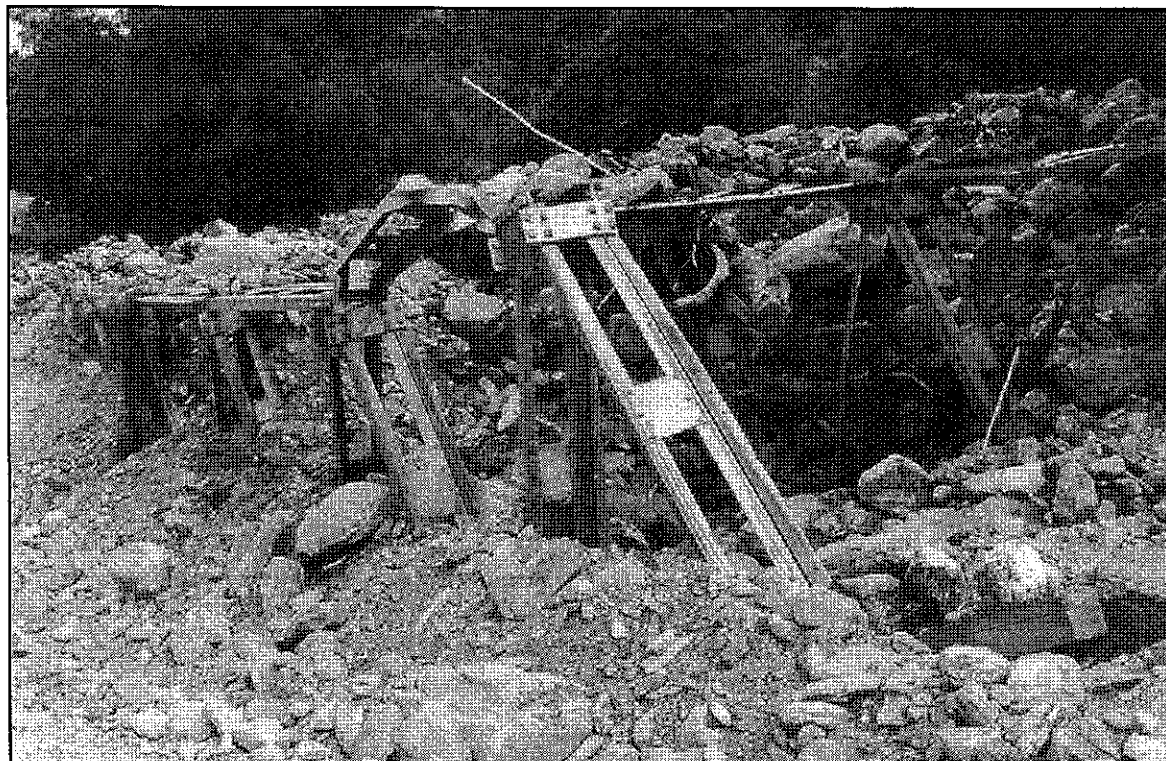
Photograph 2 Wreckage of Kowhai Creek Road Bridge Caused by January 1994 Flood
