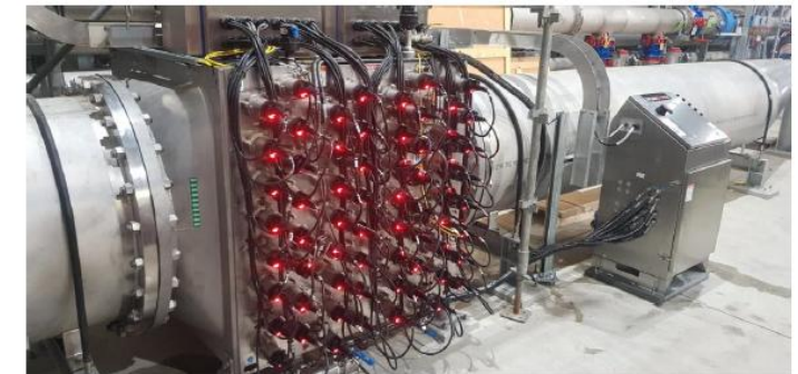
Figure 8 Example UV reactor installation (from Trojan website)
