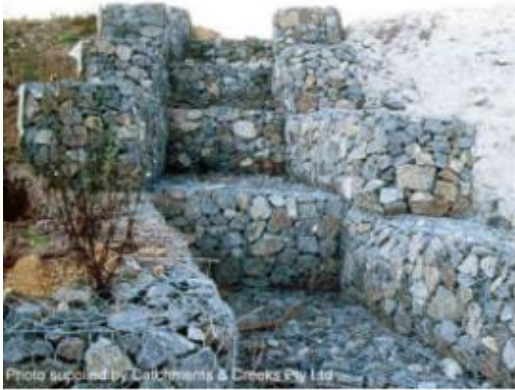
Stepped gabion chute (Qld)
