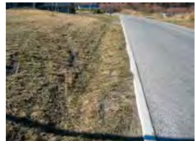
Adopt grass drainage swale and flush concrete edge to seal. Instead place concrete beneath seal edge.
