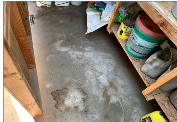
Photo 9: Chemical stains on the concrete floor of the hazardous goods shed
