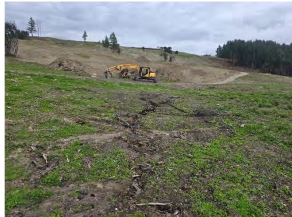
Photo 6: Lot 5 building platform marked by stake in centre. Note incipient gully erosion in front.
