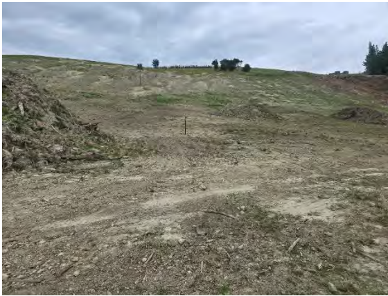
Photo 5: Lot 4 building platform marked by stake in centre. Note rear scarp of landslide at back.
